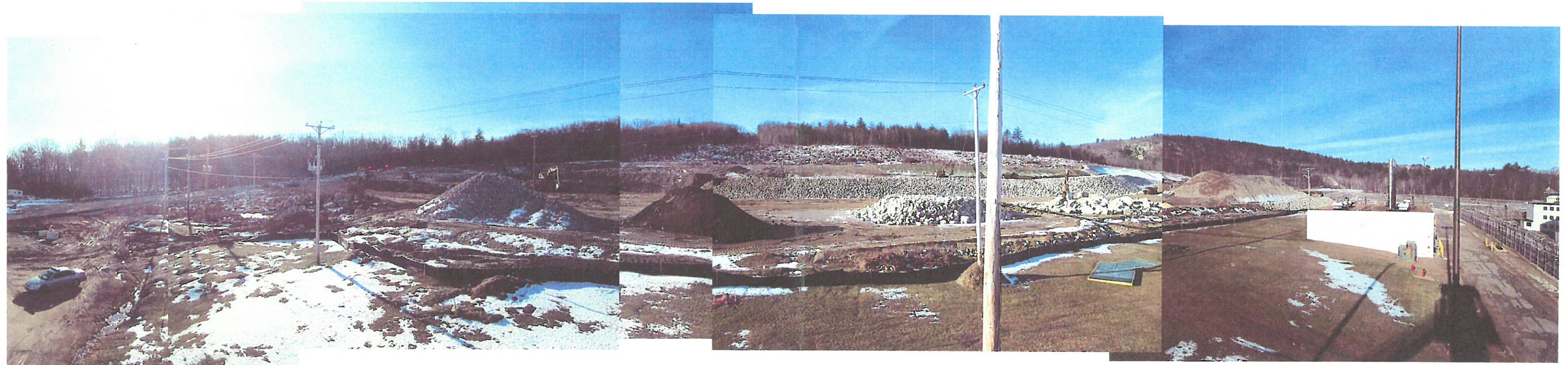
SITE FROM TOWER 1 – 12/15/2014 (GMP1 – Gilbane/Audley) NOTE: site sits fallow until 4/2016 for redesign by SMRT
