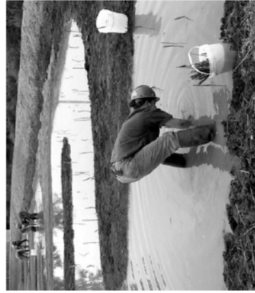
Vermont Youth Conservation Corps volunteers plant the Bartlett Brook stormwater treatment wetland.
