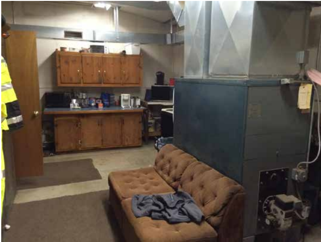
PS512 Londonderry Interior View Crew Quarters with Oil Burning Furnace
