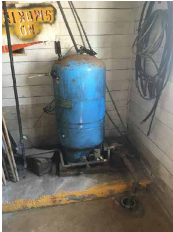
Photo-9: View of outdated and deteriorating plumbing equipment.
