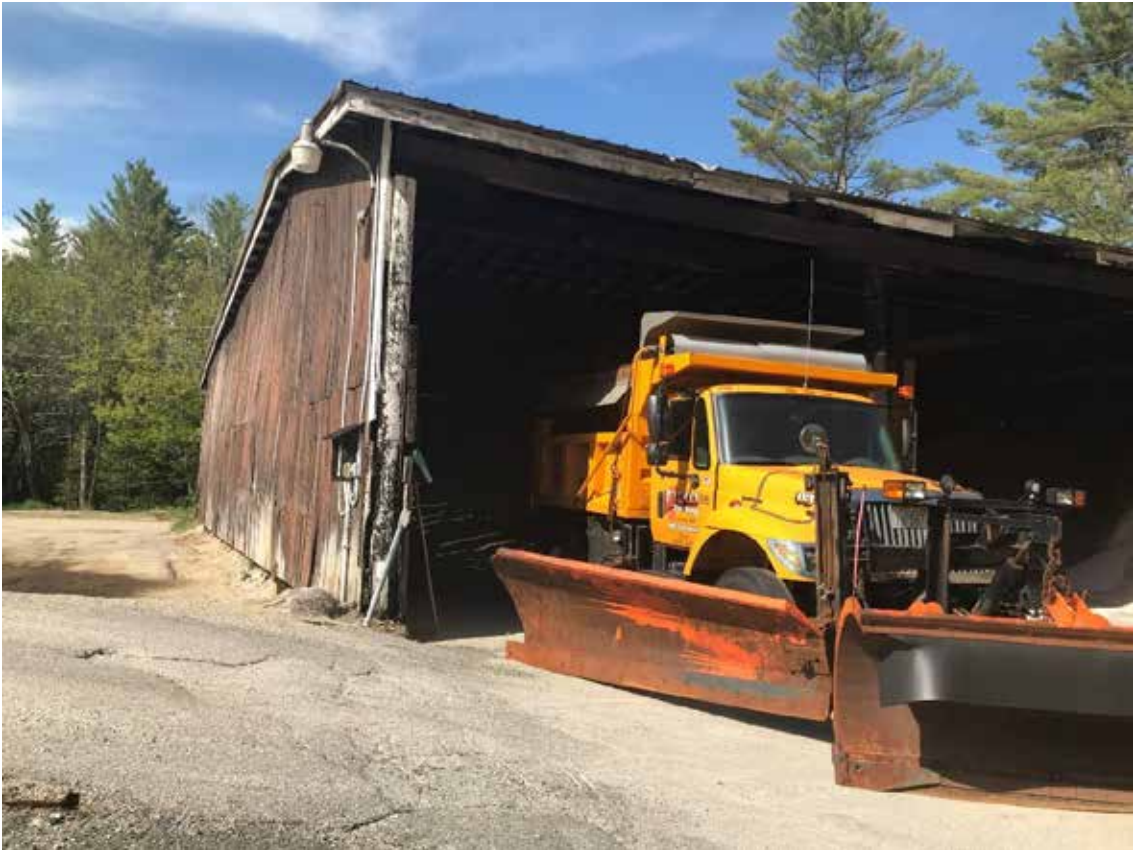
Photo 6: Lempster (215) – Salt Shed deteriorated condition
