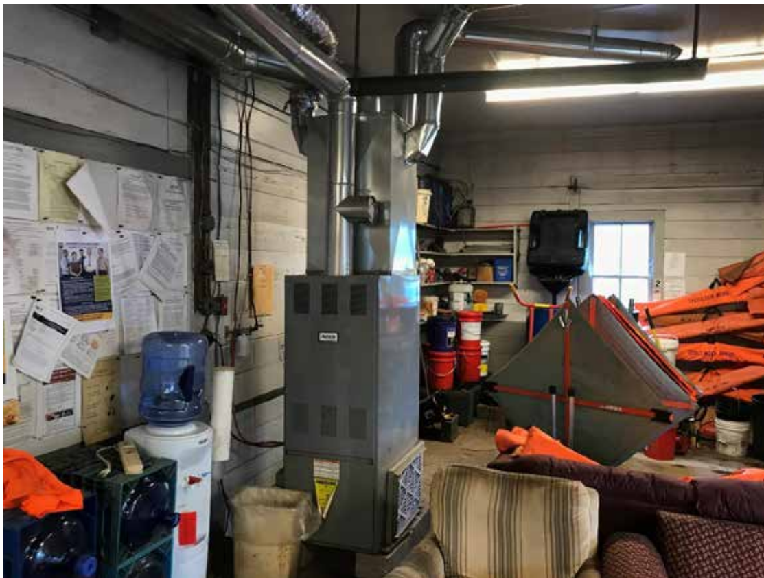
PS510 Milford Interior View garage bay with oil-fired furnace
