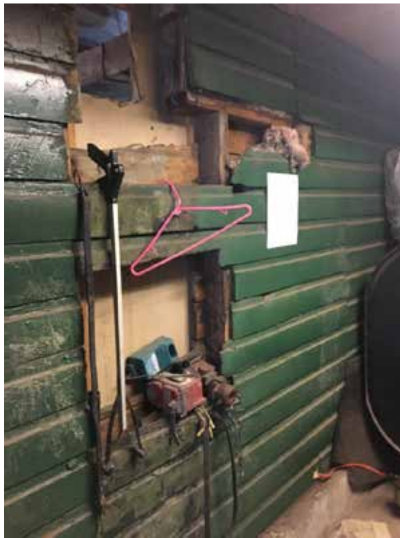
Photo-10: View of significant deterioration where portions of the original structure are exposed.
