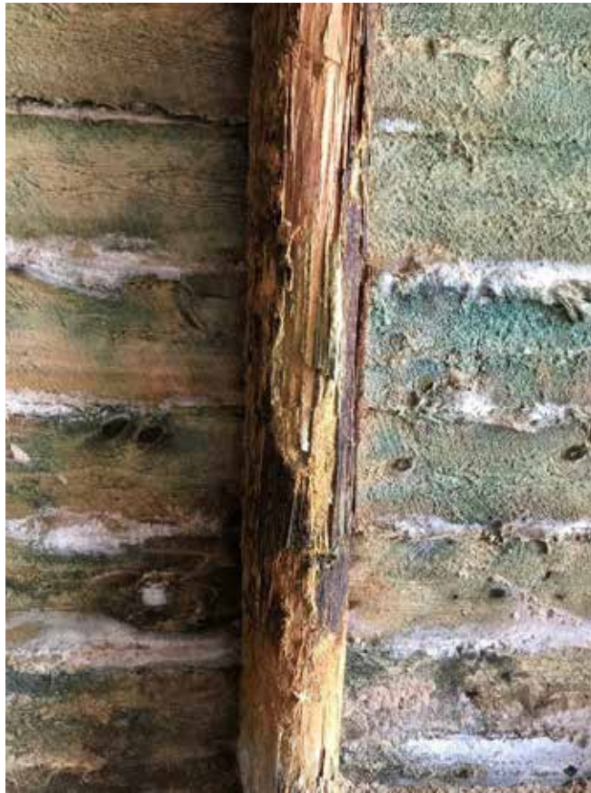
Photo 3: North Hampton – Wall and post rot
