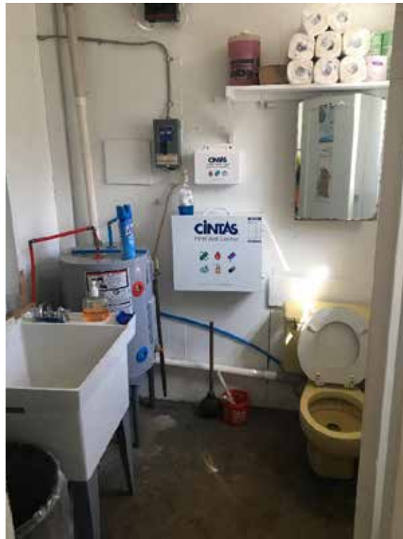
Photo-13: View of existing restroom that is non-functional due to failed septic system.
