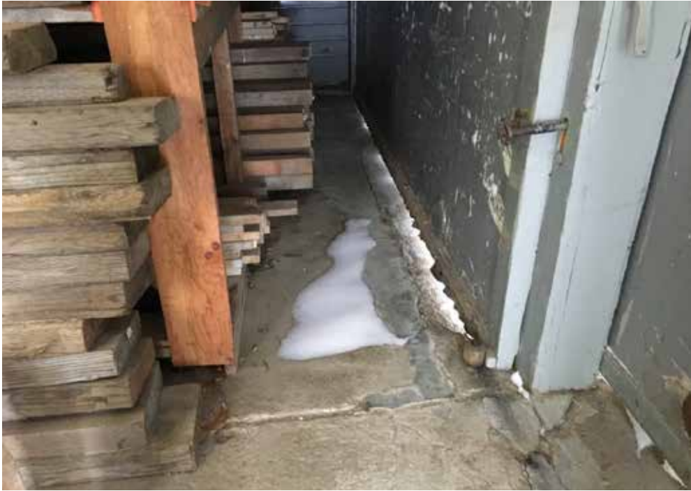
Figure 5: Interior view of area that jams sliding door
