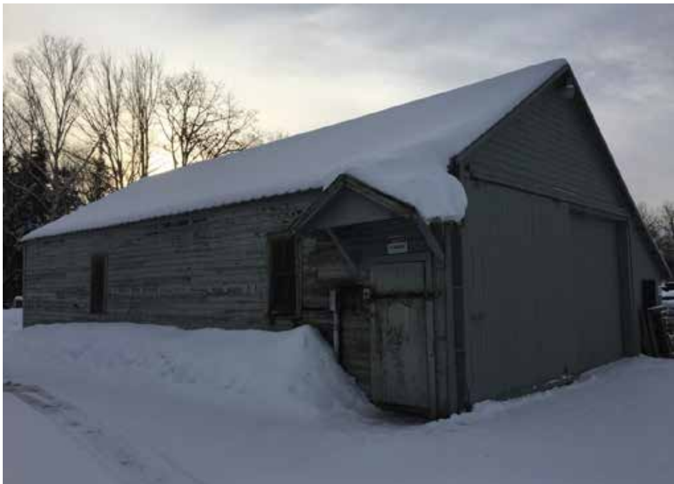
Figure 2: Sidewall in Poor Shape
