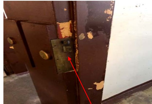
Door mechanisms worn out
