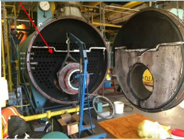
Steam tubes worn out
