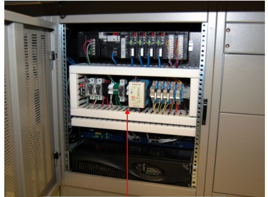
Old style door controllers
