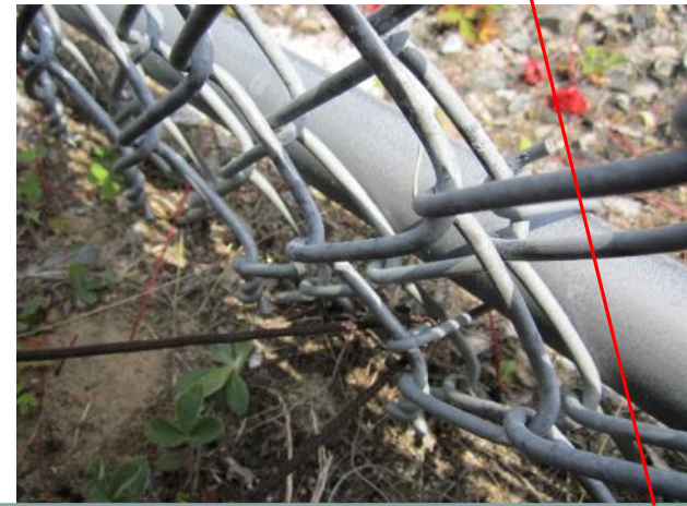
Old controllers exposed to elements
