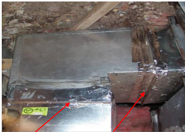
Temp repairs using tape
