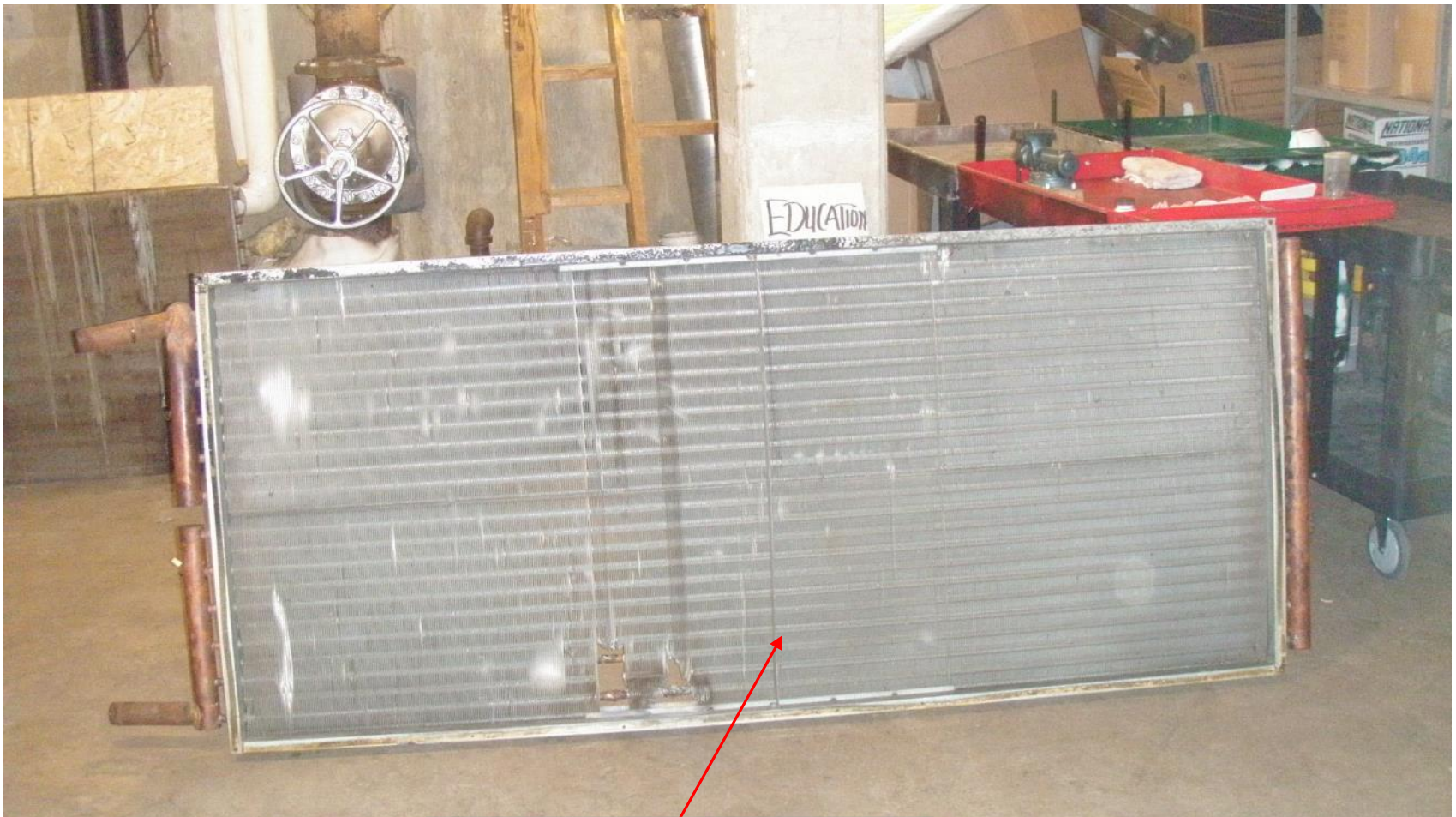
Original heating coil 1983
