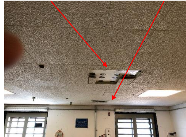
Ceiling falling down
