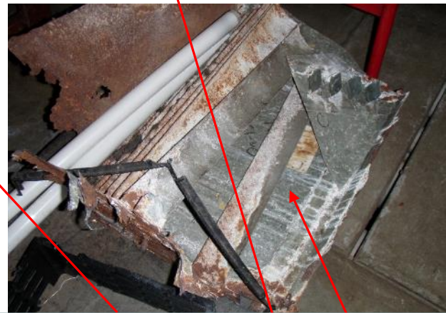
Duct work rusted through and collapsed
