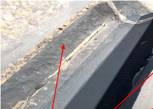
Cracks & sun damage in roof
