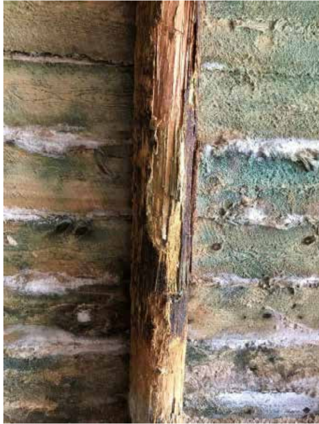
Photo 3: North Hampton – Wall and post rot
