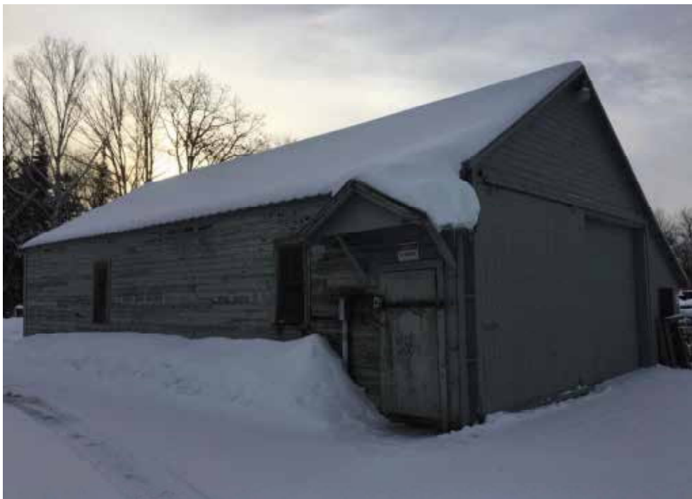
Figure 2: Sidewall in Poor Shape
