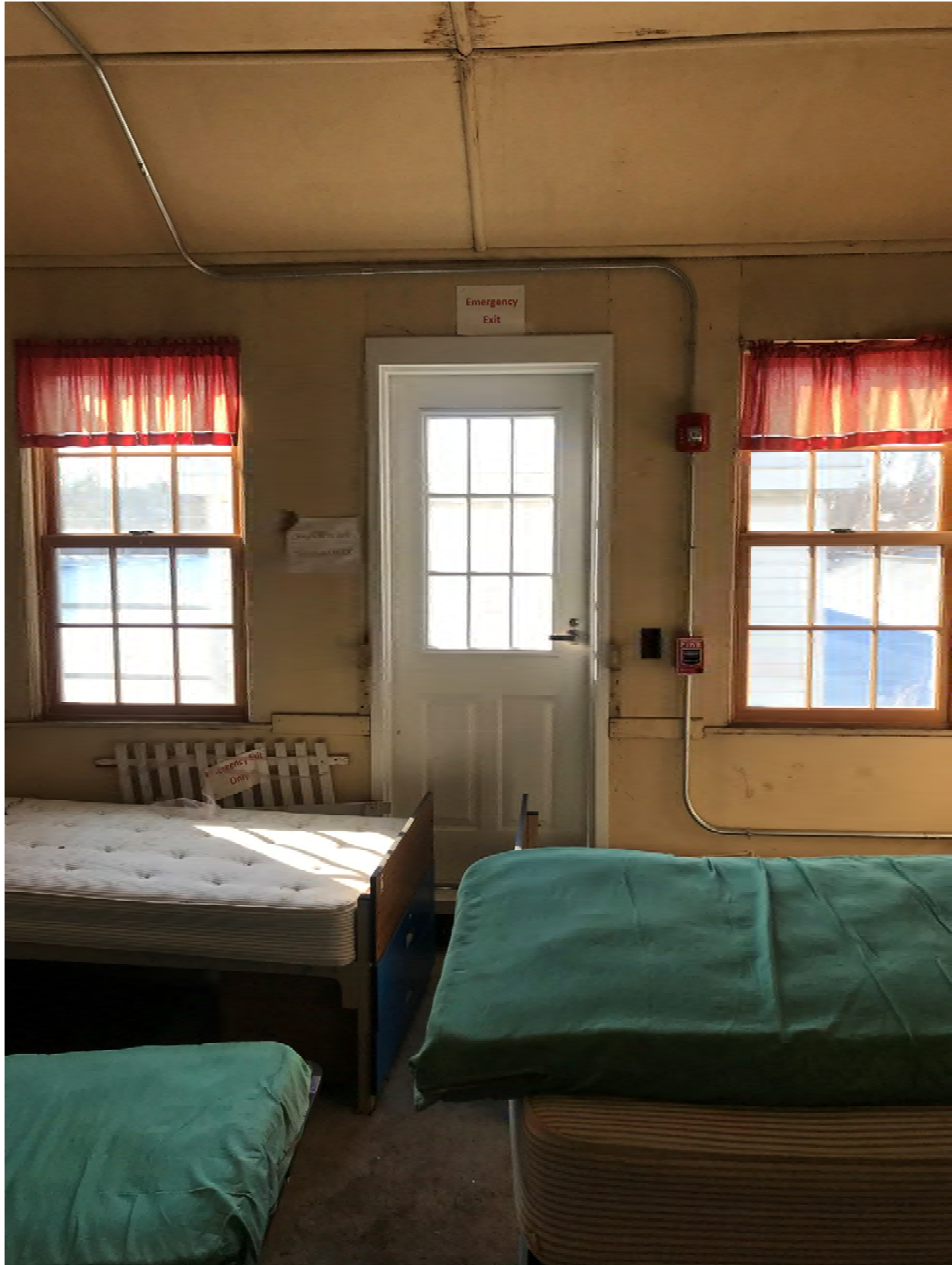
Figure 1 - Obstructed Door and Noncompliant Exit Sign
