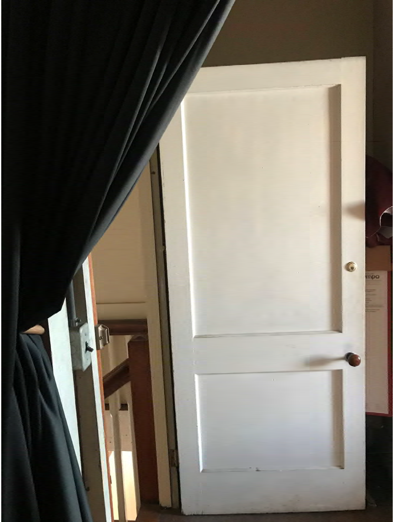
Figure 6 - Noncompliant door hardware and Unpermitted Dead Bolt
