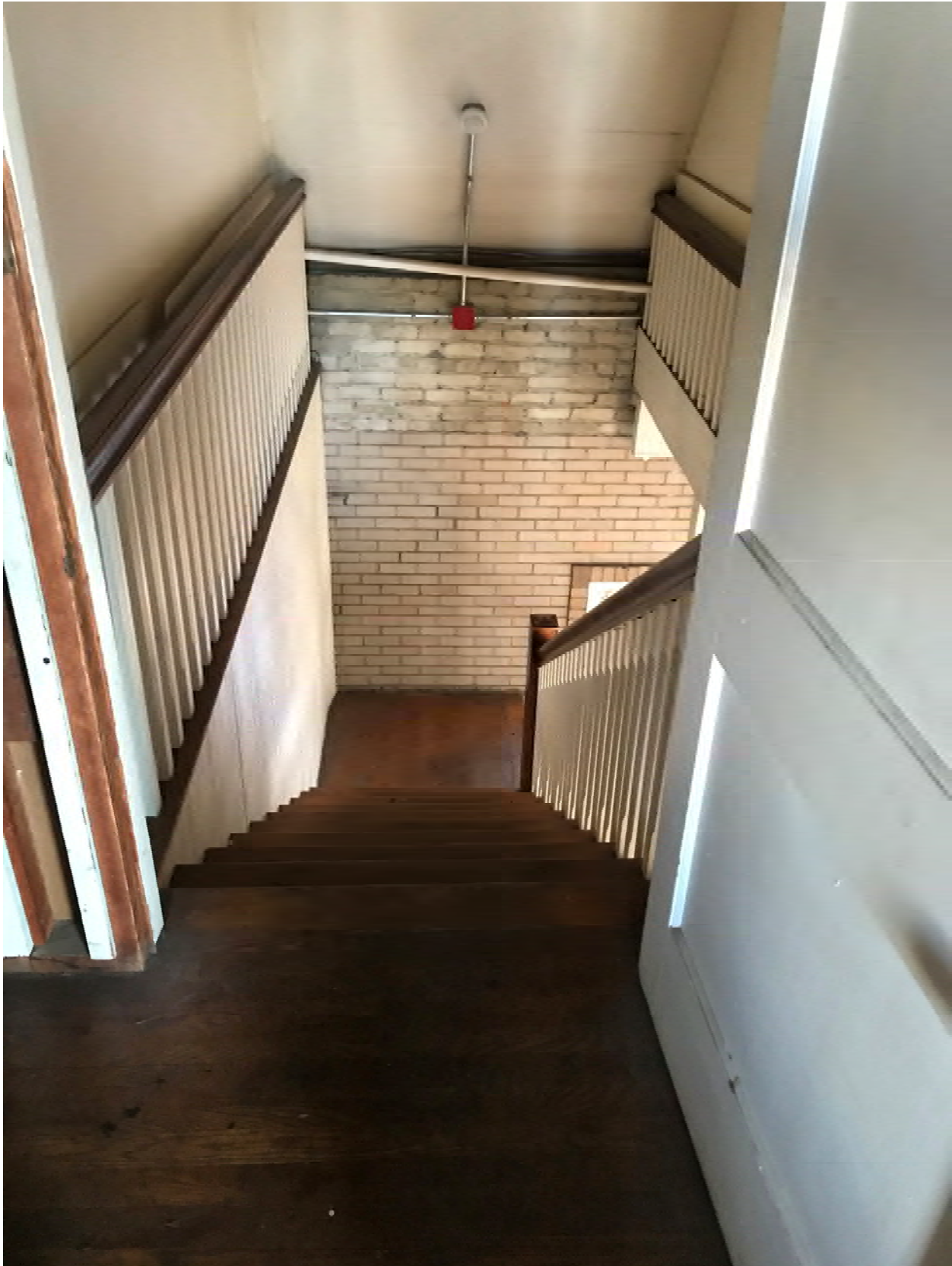
Figure 5 - Internal Stairway 1 and Enclosure which is not Smoke-Tight
