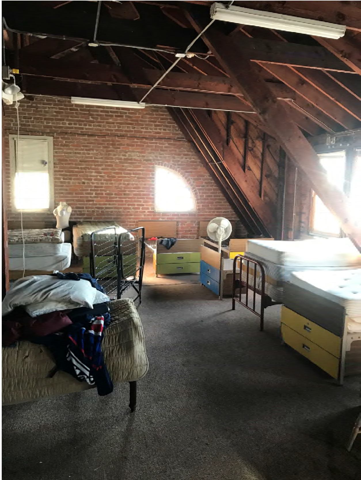
Figure 3 - Exit Aisles between Beds is Insufficient
